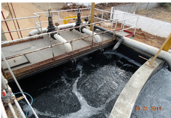
Neutralisation System /pH Correction
