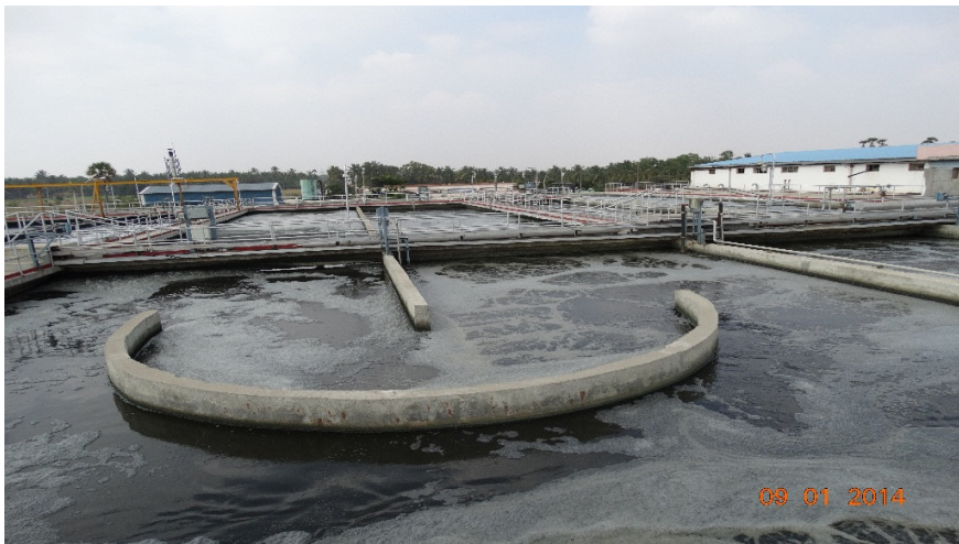
Figure 6: Secondary Treatment / Aerobic type Biological treatment system
