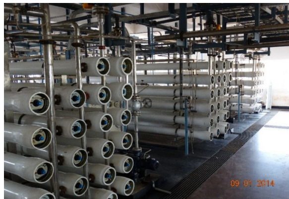
Figure 9: Reverse Osmosis plant for water recovery
