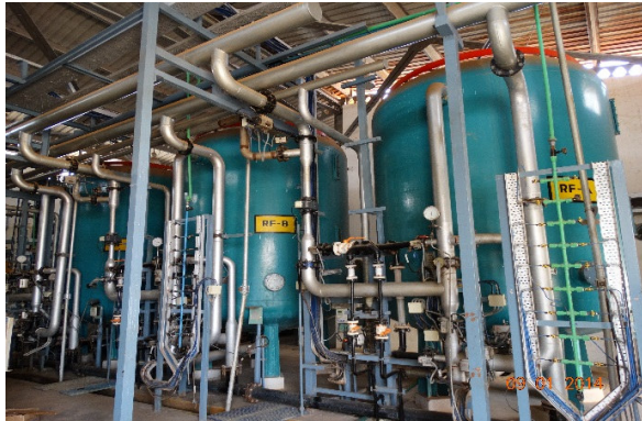
Colour removal Resin Filter
