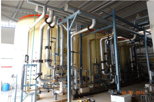
Figure 7: Typical Filtration unit
